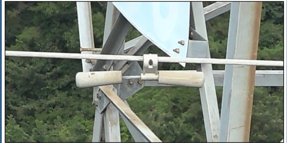
Defective SB Damper
