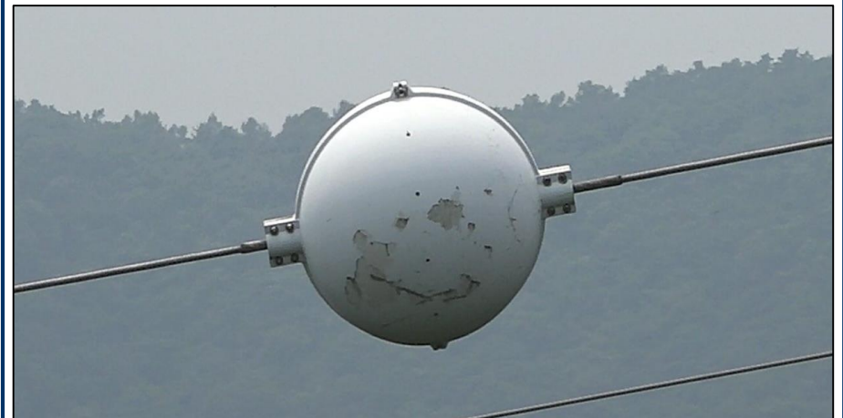
Aerial Ball Damage
