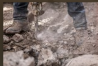
Excessive Construction Vibration Activities
