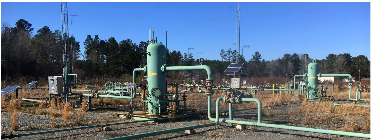
AgoraGateways automate and optimize the choke setpoint on gas wells in the Haynesville Shale.
